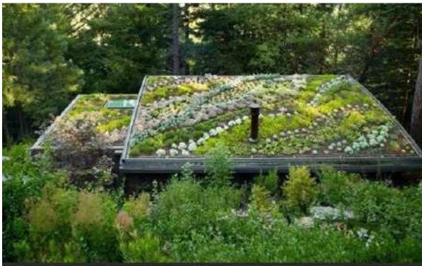
Vegetated roof slows stormwater runoff.
